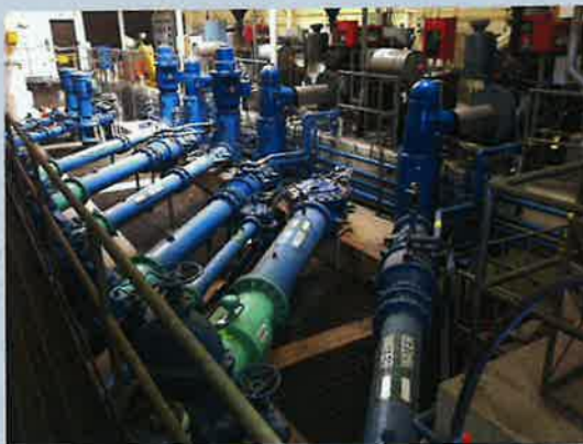
Reservoir 1 Pump Station
