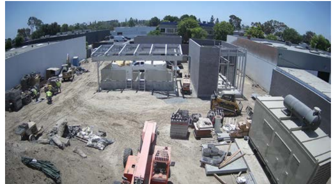
Figure 4. Well No. 12 Chemical Facility
