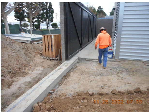
Figure 3. Well No. 14 Roller Gate
