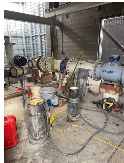
Figure 4. Well No. 14 Wellhead Piping
