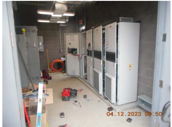
Figure 2. Well No. 12 VFD
