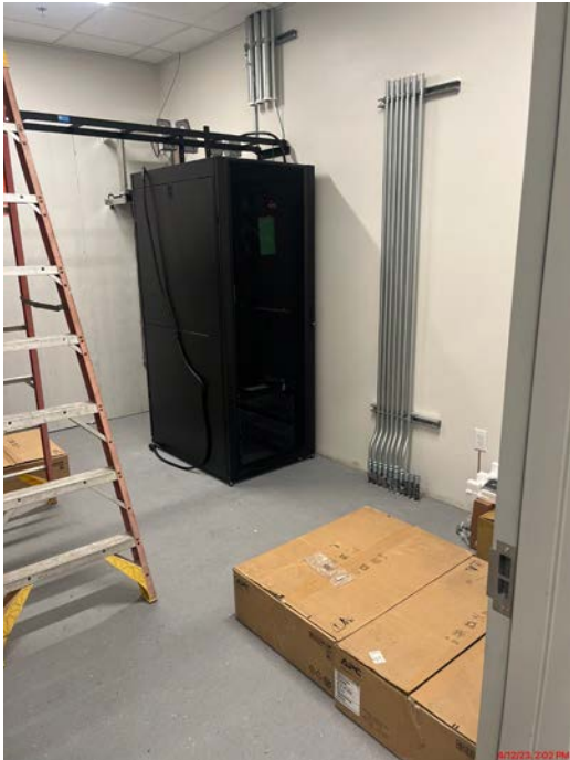
Figure 17. SCADA Server Room
