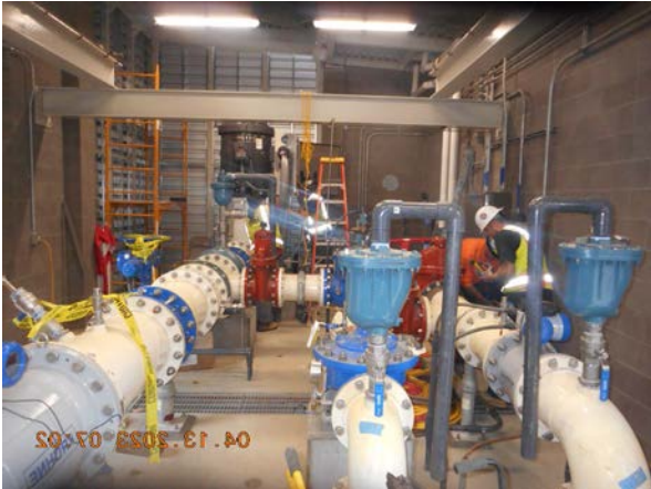
Figure 1. Well No. 14 Wellhead Piping
