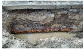
Weld seam split
