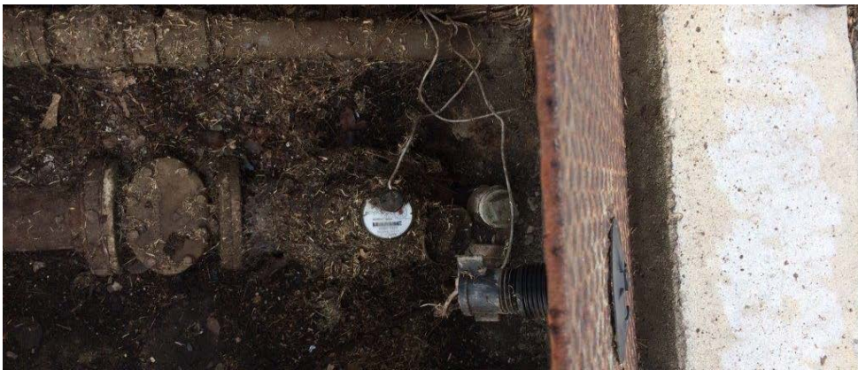
Figure 8 –TR Meter Vault
