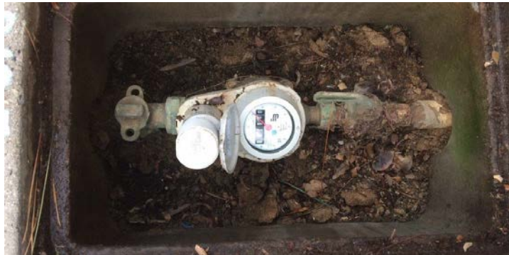
Figure 5 – Small Meter Installation w/CE Device
