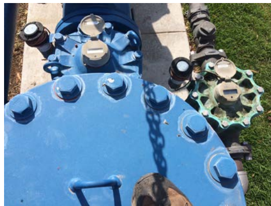
Figure 6 – Large Meter Installation w/CE/ME Device
