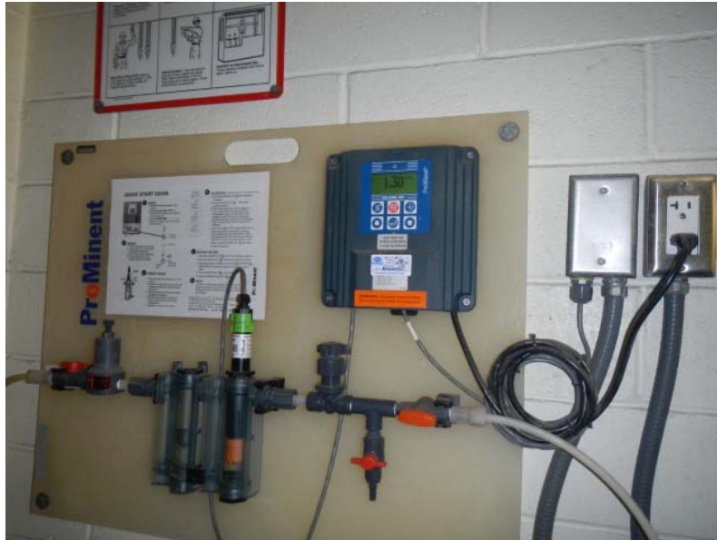
Figure 2-3. Reservoir 1 Water Quality Analyzer
