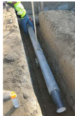
Figure 4. Underground Mechanical Piping
